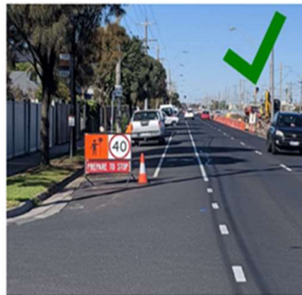
FIGURE 22: TEMPORARY SIGNAGE CORRECTLY PLACED SO NOT OBSTRUCTING CYCLE LANE
